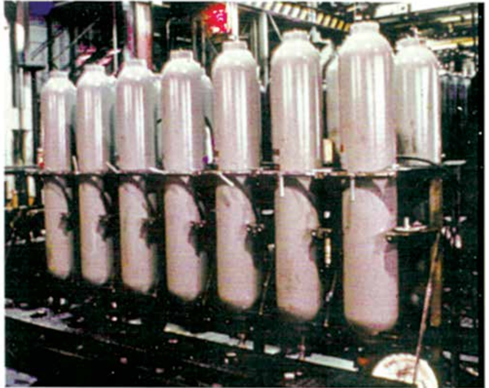
This bank of accumulators is typical of NACOL accumulator installations
